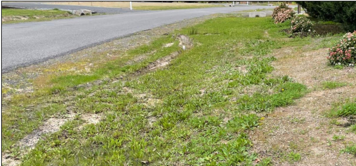
Figure 4 Typical Swale/Road Drain (Location: Golf Course Road Development)
