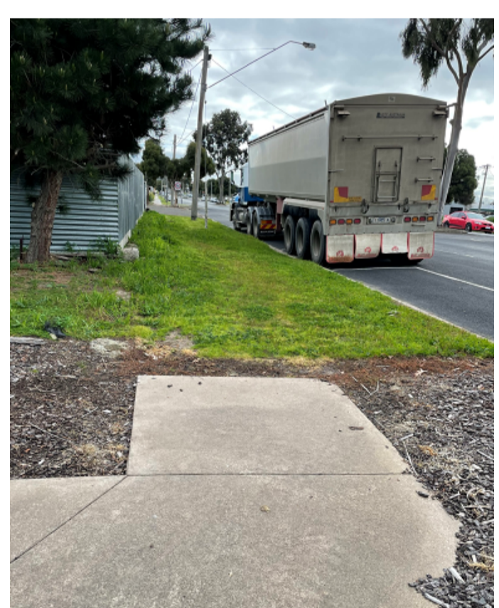
Looking north from O'Callaghans Pde showing truncation of footpath
